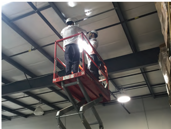
Mercmaster Connect LEDs help maintenance staff focus on larger projects, saving you time and money
